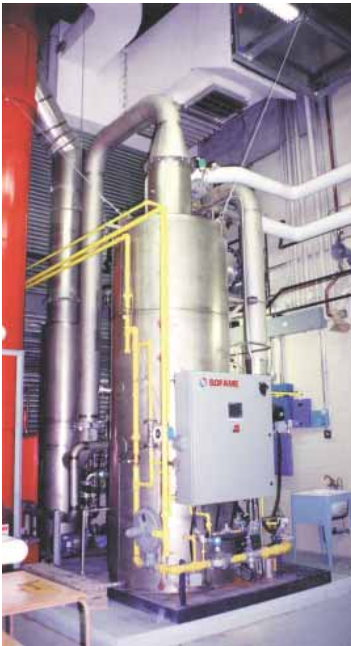
View of the 1.3 MW direct contact heat exchanger water heater.
