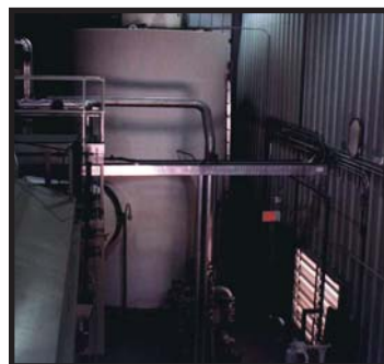
At the discharge from the economizer, a Sofame direct-contact water heater recovers 12 million Btu/hr from the flue gas, which is used to heat 300 IPGM of hot water at 120°F.
