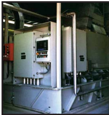
The Maple Lodge Farms 5.2 MW cogeneration unit produces 65,000 lb/hr of steam plus hot water. Its energy efficiency has been estimated at 86 per cent.
