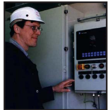
Alan Wassens, Maple Lodge Engineering/Services Manager, inspects the Allen-Bradley control panel. Wassens was a strong advocate of cogeneration for the plant. "It was a matter of finding the right fit," he says, "and rationalizing the financial investment."
