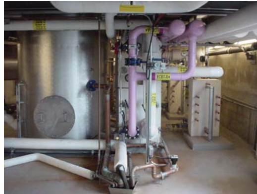
Figure 4: Flue gas plume reduction installation (direct contact economizer at left and heat plate exchangers for heat recovery of gray water at right).
